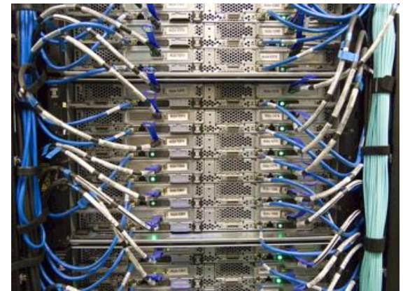
Data Center Switch
